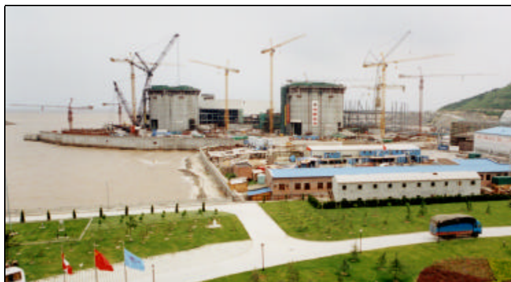
Two 728 MWe CANDU reactors at the Qinshan Phase III site in China will begin producing electricity in 2003.
